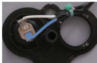
COMPRESSOR OVERLOAD (SAT)
