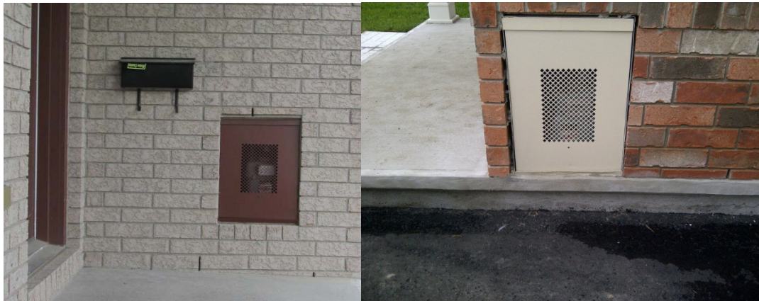
Figure 1: Examples of meter box service installations in the Ottawa area.
