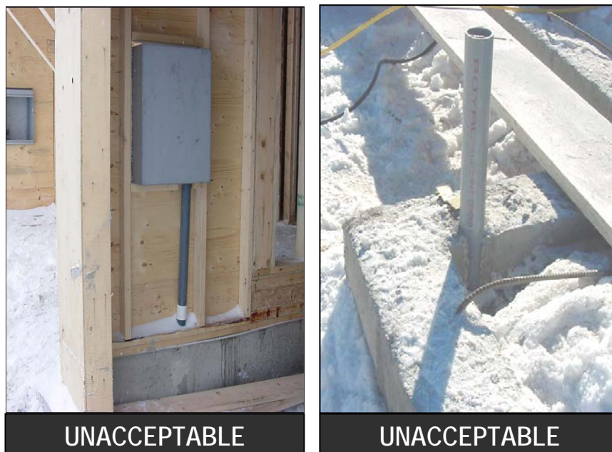
Figure 3: Examples of common pitfalls and unacceptable installations of the PVC conduit.
