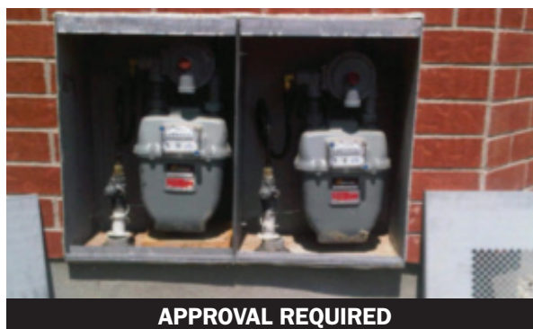
Figure 5: Two Meter Boxes Side-by-side - Approval from Enbridge Gas Distribution is required during the architectural design stage prior to installation.
