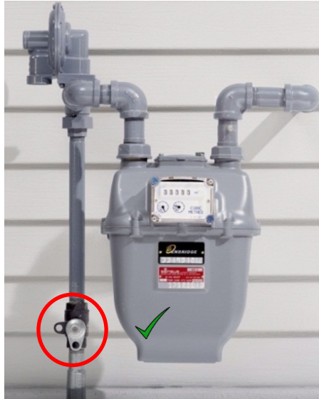
Figure 3: Service valve on a small residential building.
