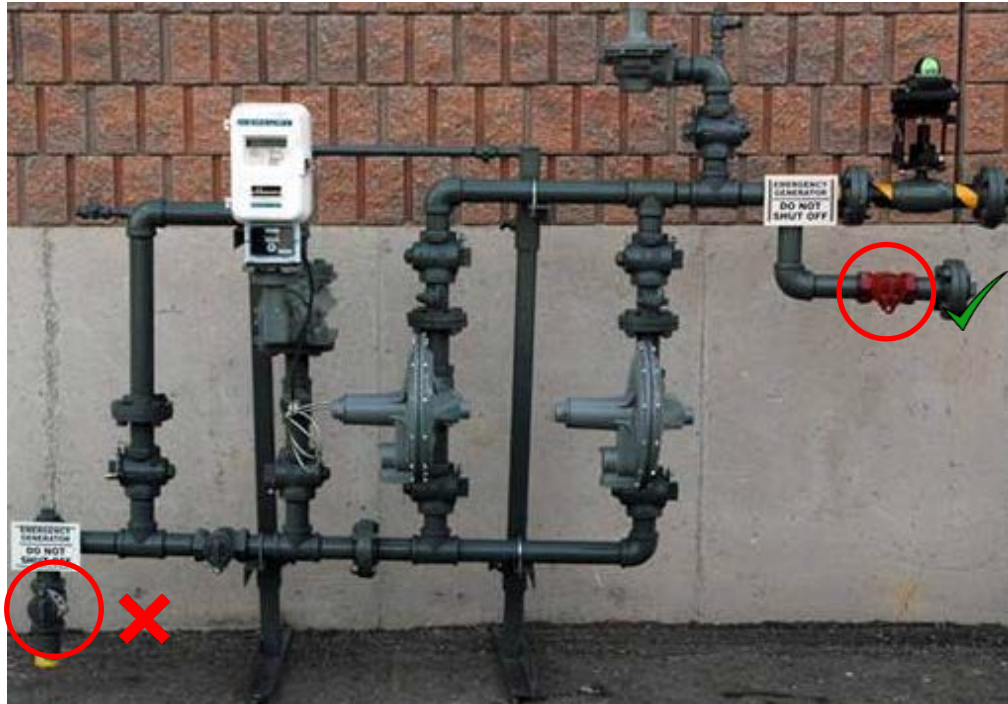
Figure 5: Gas pipe system with a Life-safety Emergency Generator supply line
