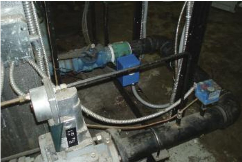
Variance-approved modification to a boiler.
