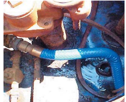
Piping Over Bent
