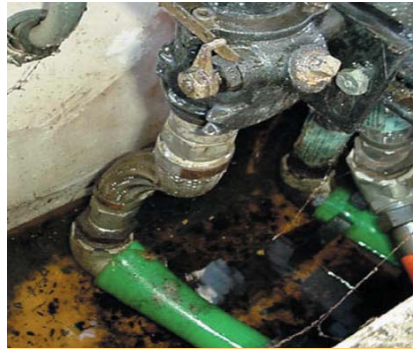
Fittings/Flex Connectors Twisted/Misaligned
