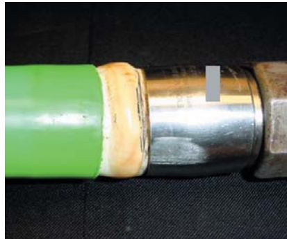
Pipe Swelling and Bulging
